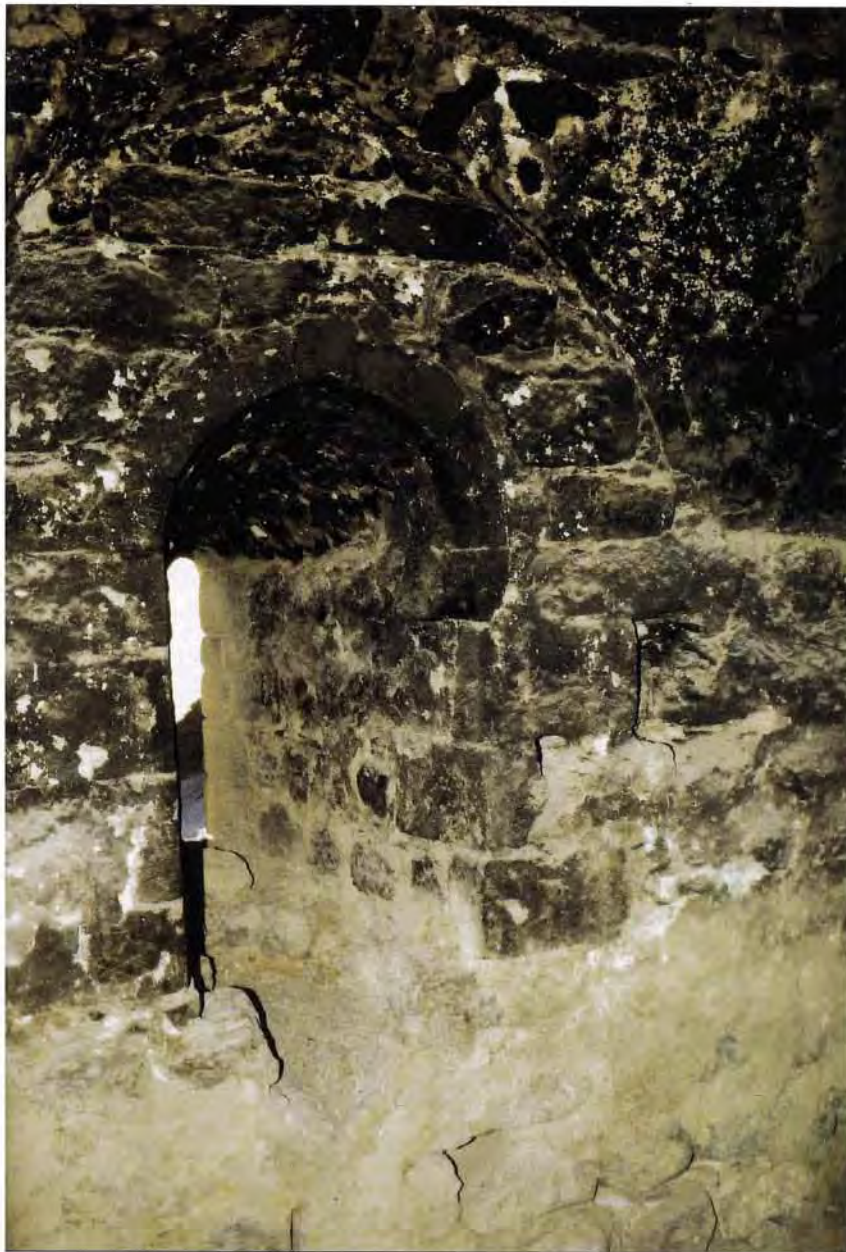
An embrasure in the largest surviving tower at Le Vaux Moise (al-Wu'aira) castle. Some features at al-Wu'aira are particularly important because they provide early examples of Crusader military architecture in a castle that was then abandoned, rather than being altered following the Islamic reconquest.
